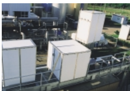
Setting up of two Banquise® systems and one Cascade® system on the chilled water tanks
